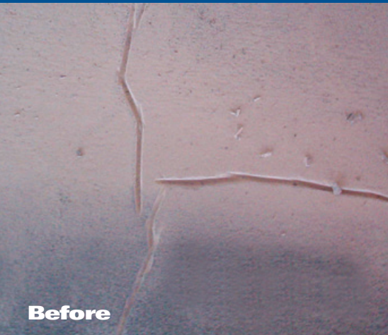
Narrow concrete cracks before filling with FastPatch LV.
